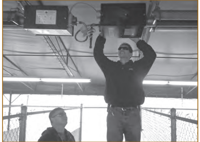
Wally Watkins and Paul Cano work to convert the system from propane to natural gas.
