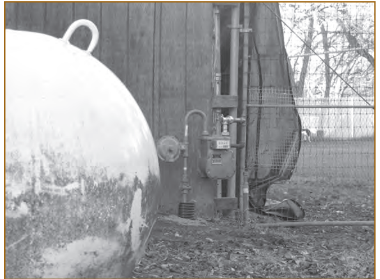
The old propane tank (left) was phased out by a new gas meter, thanks to the efforts of RHT Energy Solutions and Avista.
